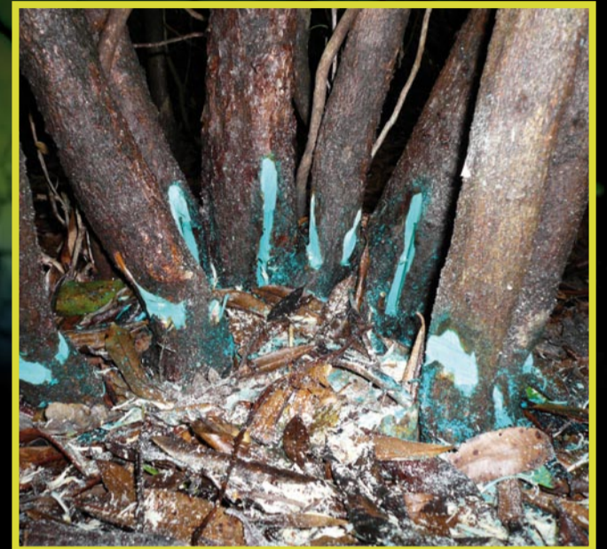
ALTERNATIVELY TREAT MULTI-STEMMED PLANTS WITH LESS ACCESSIBLE BASES BY APPLYING CUTS TO EACH STEM AS SHOWN ABOVE.
